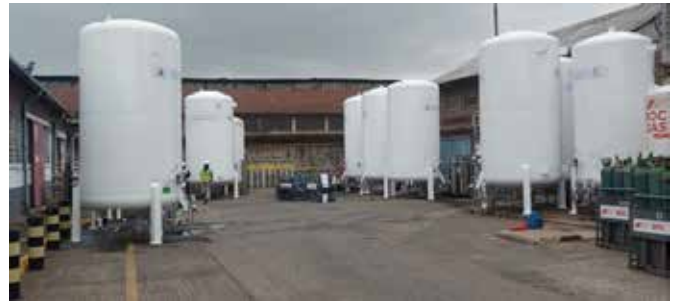
The tanks at BOC KENYA PLC Nairobi site.
